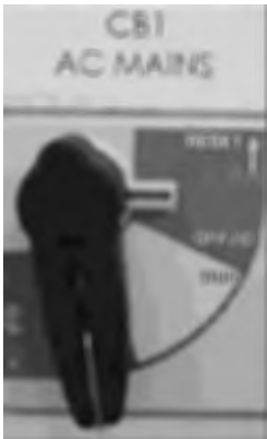
AC Mains Circuit Breaker
