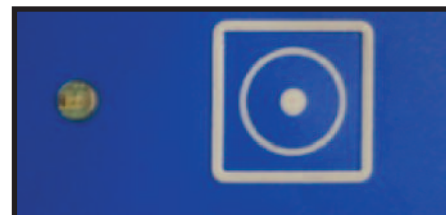
Figure 16.2-3: System Power On Push Button found on the control panel at the Operator's Console
