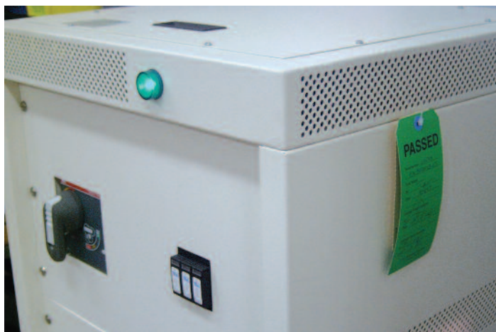
Figure 6.4-1: Isolation Transformer is receiving power
